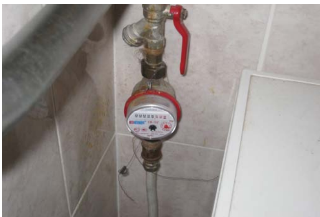
On the photo: water meter that was installed in Olga Senova's house
