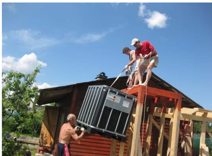
On the photo: process of solar water heater installation at the country cottage
